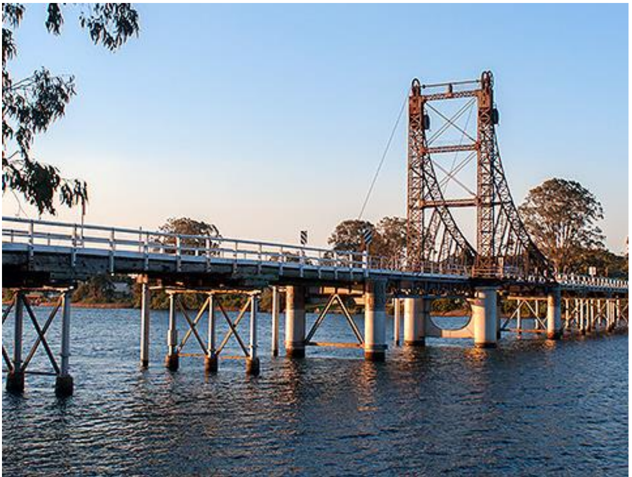
McFarlane Bridge, spanning the Clarence River to connect Maclean and Woodford island
